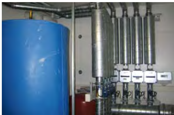
Fig. 2: The GGH company in Heidelberg has implemented a zero-emission concept prepared by the planner, “solares bauen GmbH”, in renovating its “Blaue Heimat” building. The combined heat and power (CHP) plant, together with a buffer storage tank, meets 95 % of the building’s demand for heating energy.
