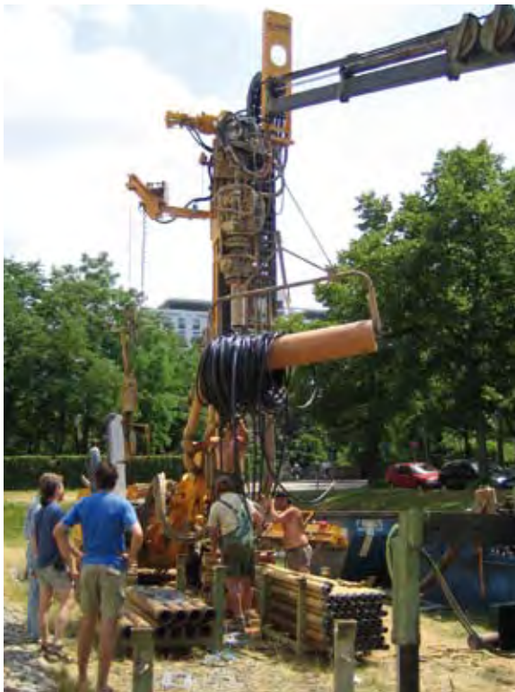
Fig. 1: Installation of three underground pipes, each reaching a depth of 80 m, in front of the Fraunhofer ISE premises. In summer, the underground loop is used for heat rejection for a solar-thermally driven adsorption chiller with about 15 kW of thermal power for re-cooling (Fig. 2). In winter, the underground pipes supply low-temperature heat for heat-pump operation of the same machine.
