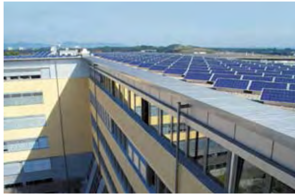
Fig. 1: PV system on the Solar Info Center in Freiburg: The 50 kWp system, which was installed in 2003, has consistently delivered optimal yields since then.
