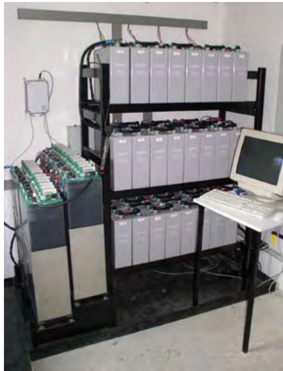
Fig. 1: Three of the four battery strings installed at the Rappenecker Hof. The implemented battery management system is able to determine the state of the batteries accurately (charge, aging), apply optimised charging strategies and react flexibly to consumer behaviour and generator performance. This is achieved by dividing the storage unit into several parallel strings, which can be connected independently of each other.
