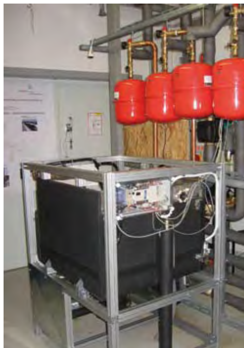
Fig. 2: Adsorption chiller with a heat-pump function. The rated cooling power amounts to 5.5 kW. The input air for the kitchen of the Institute canteen is cooled with this plant. The driving heat is supplied by flat-plate collectors with an area of 22 m 2 and by the heating circuit of the Institute. The plant was developed by the SorTech company, a spin-off from Fraunhofer ISE, with the support of the Institute.
