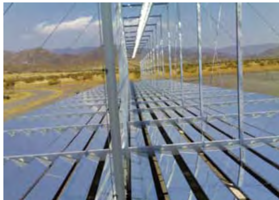
Fig. 2: Demonstration collector in Almería. The hydraulic connection of the collector to the direct evaporation trough is variable, so that different operating conditions of the collector (pre-heating, evaporation and overheating) can be investigated without difficulty.
