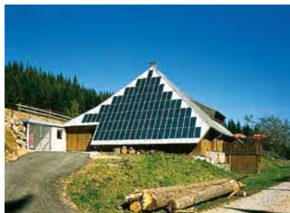
Fig. 2: The hybrid system at the Rappenecker Hof consists of a PV generator with 3.8 kWp, a fuel cell with 1.2 kW, a wind energy converter with 1 kW, a diesel generator with 9.6 kW and a battery storage unit with a capacity of 62 kWh. Within a field test, we are subjecting the battery management system that we have developed to the real operating conditions at the Rappenecker Hof.
