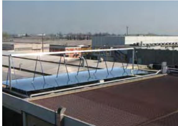
Fig. 1: Fresnel collector from the Freiburg company, PSE GmbH. The collector is used in Bergamo, Italy for a cooling application (NH 3 /H 2 O absorption chiller). The construction with the primary reflectors lying parallel to the roof means that the collector offers little wind resistance, so that it can easily be integrated into the building structure.
